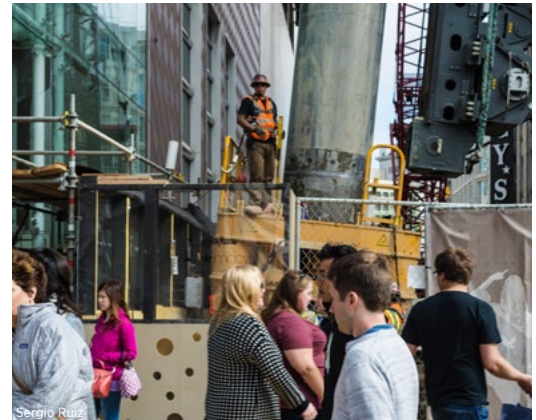
This photo shows the construction of the Central Subway in San Francisco along Stockton Street near Union Square. Over 60 percent of the funding for the $1.6 billion transportation project comes from the federal government. 45 In the future, regional transportation projects may have to rely more on local and regional sources of funding. ▲
